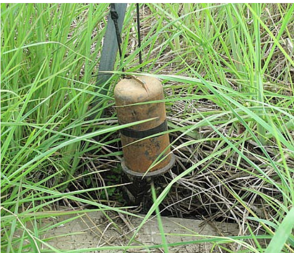
The phone cable connector in Cullen Road (our own phone line) lifted out of the pit and hung out to dry on a star picket!
