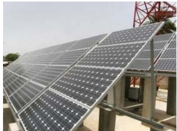
Huawei Solar Power Base Station
